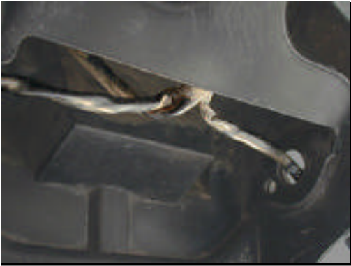
Figure 4.2 Wiring under rear tail light
